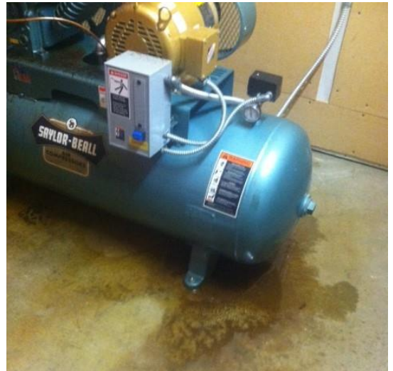
FIGURE 1 – NORMAL OIL DISCHARGE ON FLOOR
